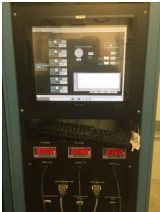
Hall B Gas Shed • DC Gas Mixing and Regional Supply
